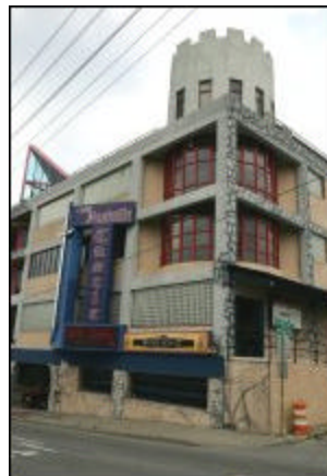
This downtown building, located at 300 Second Ave. S. and known as The Castle, is being given an exterior overhaul as it transitions toward The Gateway Entertainment Complex. Photo by Anthony Estes
